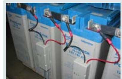
Figure 10: BCM's Installed on 12V Battery Blocks
